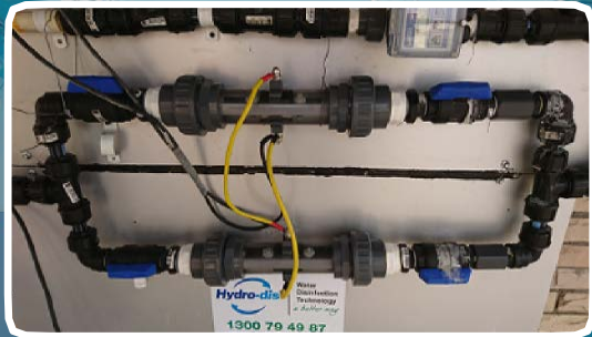
Gen 4 cells installed
