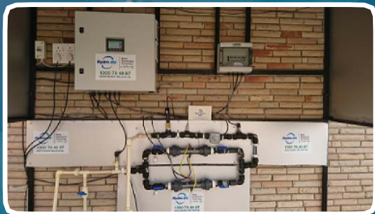
The Demonstration Unit installed at MNIT
